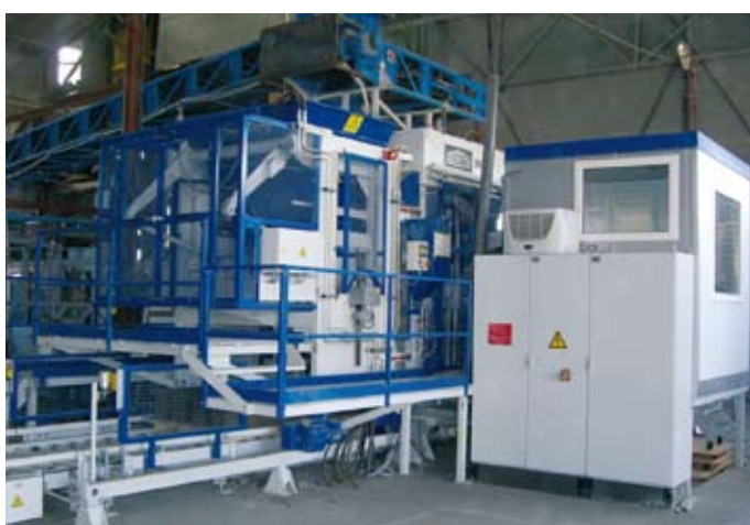
Fig. 3: Zenith 844 multilayer machine with soundproof control room.
